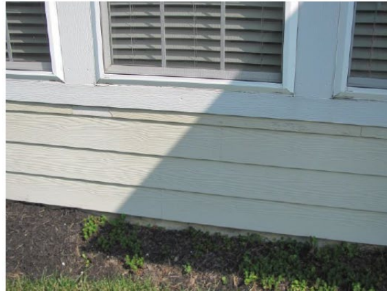
Sealant deterioration and peeling finish at fiber cement, Unit 100
